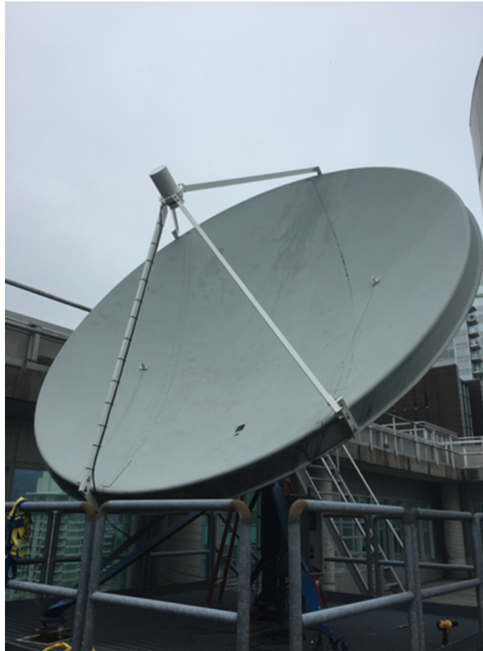
Figure 1 GOES-R Satellite Reception Antenna (reflector dish)
