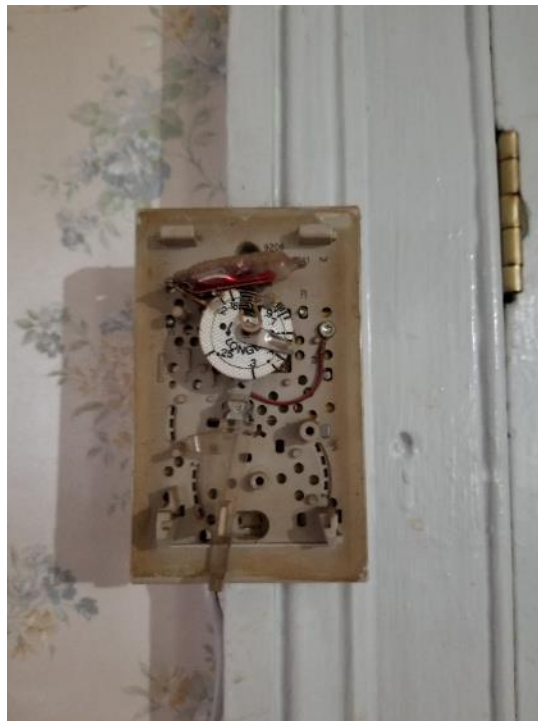
Photo 8: View of mercury-containing thermostat in the first floor kitchen.
