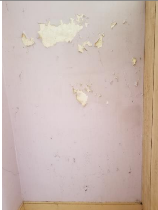
Photo 5: View of the lilac lead-based paint on the second floor washroom walls.
