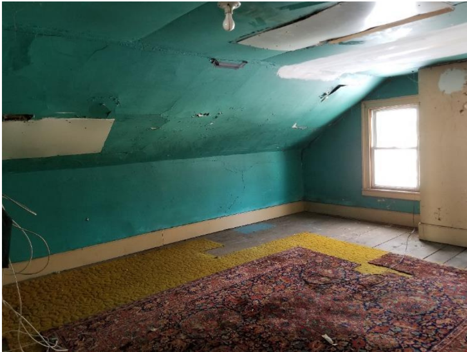
Photo 2: View of the teal lead-based paint in the second floor office.
