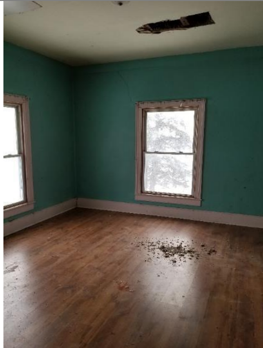
Photo 7: View of pink lead-based paint on second floor bedroom 3 window frame and trim.
