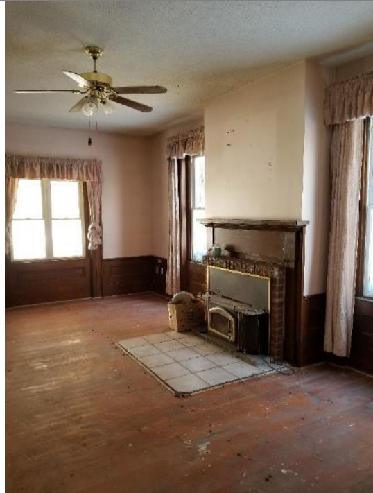
Photo 3: View of the brown lead-based paint on the first floor living room moulding and trim.
