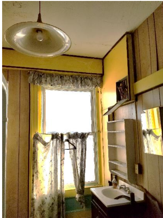
Photo 4: View of the yellow lead-based paint on the first floor washroom trim.
