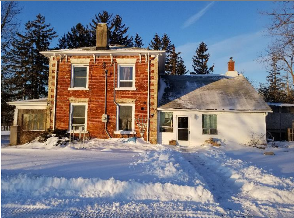
Photo 1: View of the exterior of the subject building and suspected ACM roofing materials.
