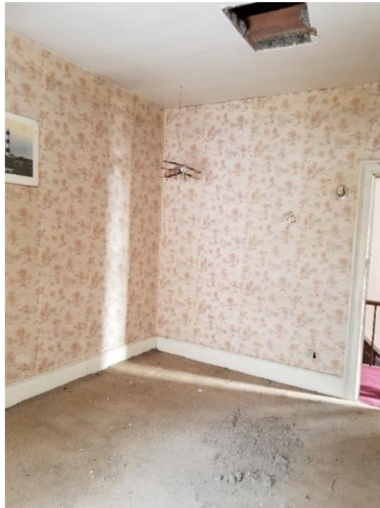
Photo 6: View of the second floor bedroom 1 carpet under which there is brown lead-based paint on the wood floors.
