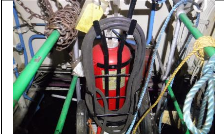
13. CO2, water and dry chemical fire extinguishers noted.
