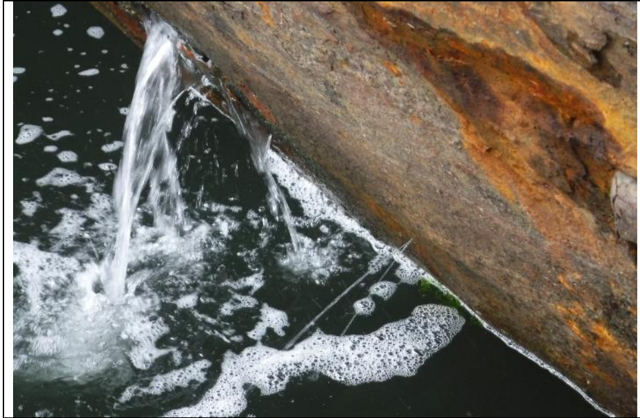
3. Port fed hull section – breach
