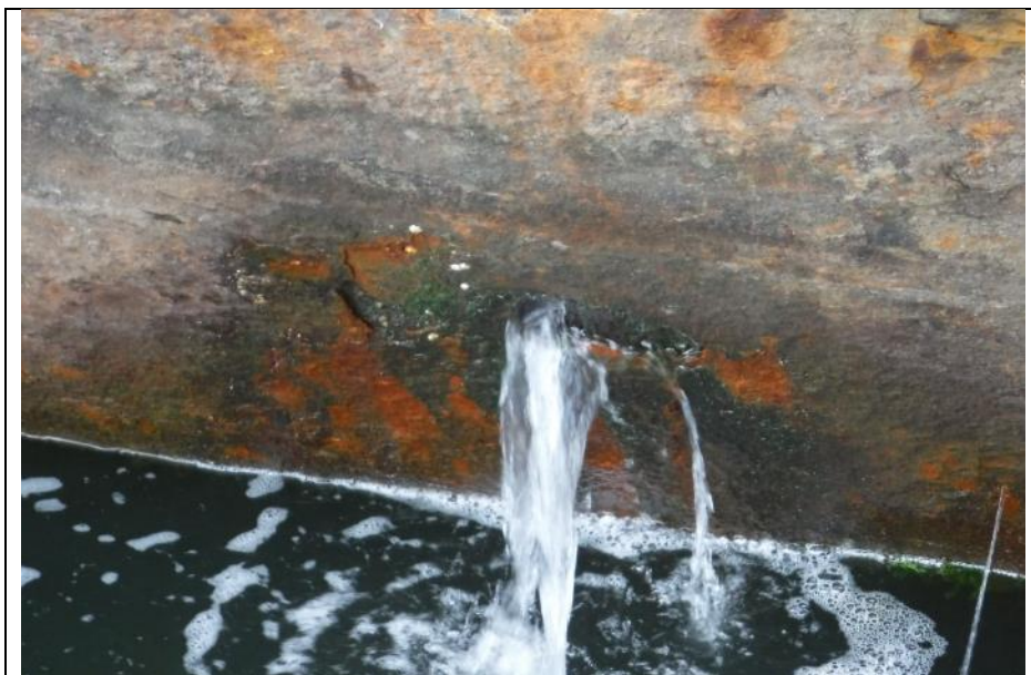
2. Port fed hull section – breach
