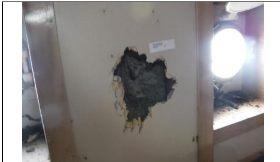
10. Insulation behind cladding in messroom area containing asbestos.
