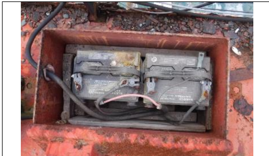
2. Lead batteries on wheelhouse deck.
