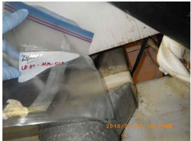
Photo 42. Sample locations LB-B4-ACM-01A-C; duct insulation. Confirmed asbestos-containing material (50% Chrysotile).
