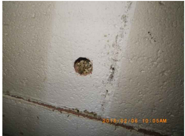
Photo 110. Pre-existing hole in cinder block wall inside the Dry Storage.
