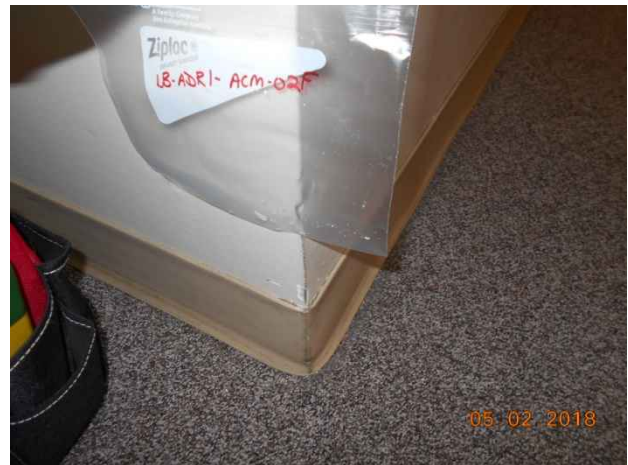
Photo 8. Sample location LB-ADRI-ACM-02F; drywall mud joint compound in hallway near R.107.
