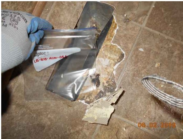
Photo 93. Sample locations LB-B18-ACM-06A to C; grey-red floor tile and fibrous mix in bathroom (third layer). Confirmed asbestos-containing material (30% Chrysotile).
