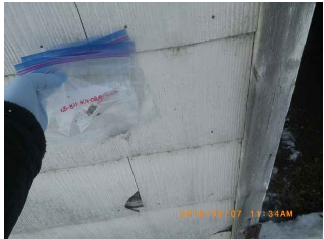
Photo 70. Sample locations LB-B11-ACM-02A to C; exterior wall board. Confirmed asbestos-containing material (25% Chrysotile).
