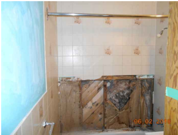
Photo 81. Damaged wall with visible mould on insulation inside bathroom.
