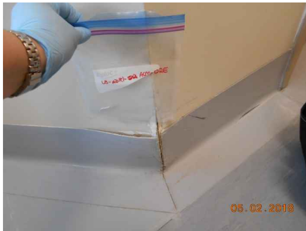
Photo 7. Sample location LB-ADRI-ACM-02E; drywall mud joint compound in hallway near R.170.
