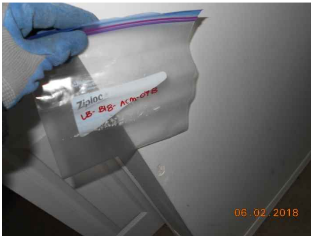
Photo 95. Sample location LB-B18-ACM-07B; drywall mud joint compound in basement rear bedroom.
