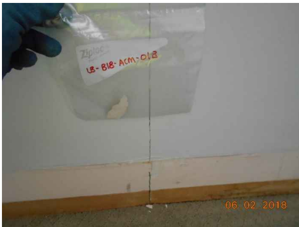
Photo 83. Sample location LB-B18-ACM-01B; drywall mud joint compound from upstairs wall. Confirmed asbestos-containing material (1% Chrysotile).
