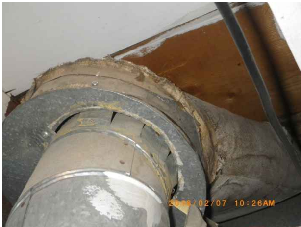
Photo 41. View of ducting in the basement.
