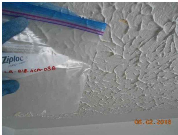
Photo 89. Sample location LB-B18-ACM-03B; textured ceiling plaster from living room (sample not analyzed based on confirmed asbestos in sample LB-B18-ACM-03A).
