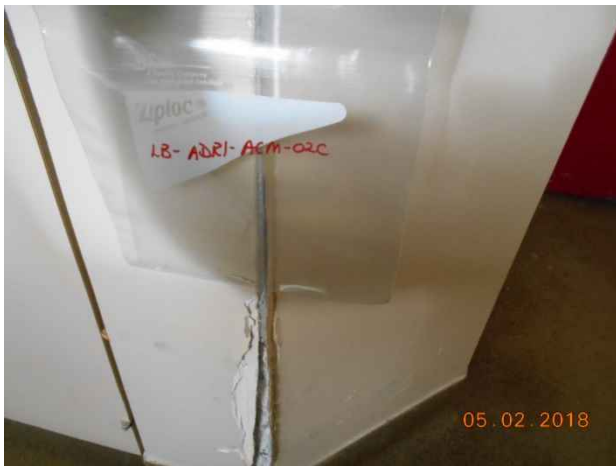
Photo 5. Sample location LB-ADRI-ACM-02C; drywall mud joint compound in hallway near R.402.
