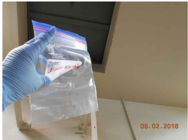
Photo 6. Sample location LB-ADRI-ACM-02D; drywall mud joint compound in R.427.
