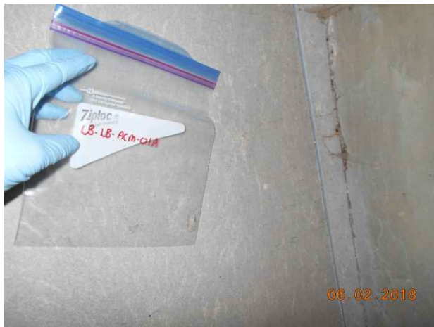
Photo 73. Sample locations LB-LB-ACM-01A to C; cement board in mechanical room. Confirmed asbestos-containing material (30% Chrysotile – Transite).
