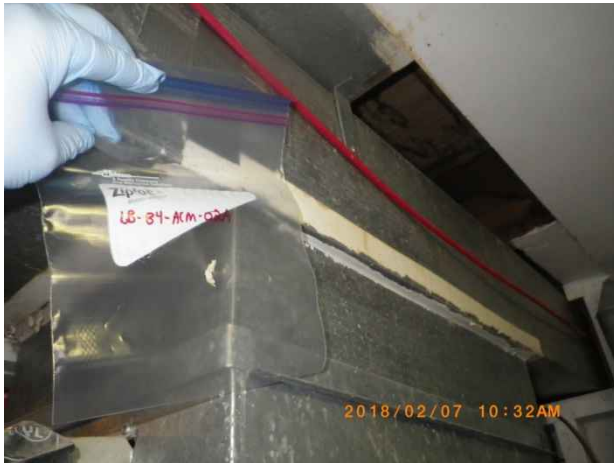
Photo 43. Sample location LB-B4-ACM-02A; paper-wrap around ducting. Confirmed asbestos-containing material (50% Chrysotile).
