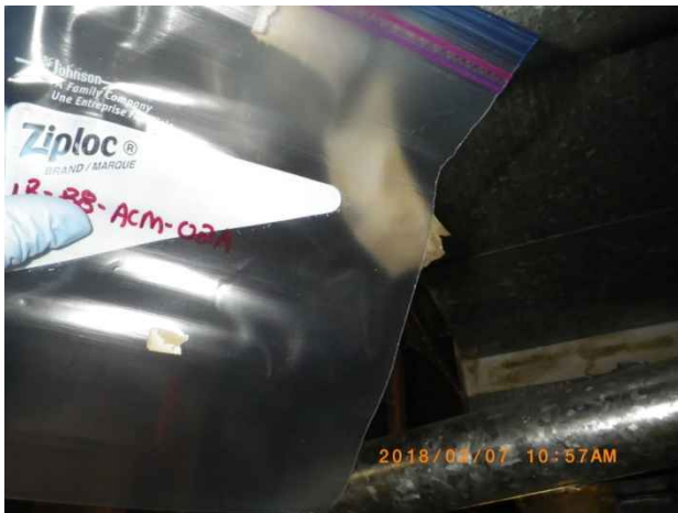
Photo 65. Sample location LB-B8-ACM-02A; paper-wrap around ducting. Confirmed asbestos-containing material (50% Chrysotile).
