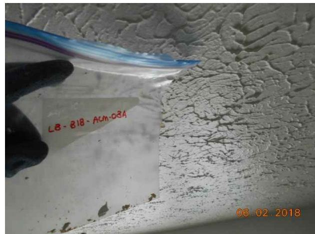
Photo 88. Sample location LB-B18-ACM-03A; textured ceiling plaster from living room. Confirmed asbestos-containing material (1% Chrysotile).
