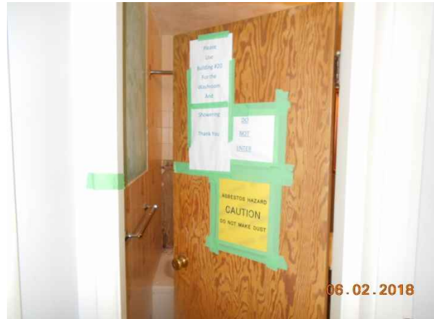
Photo 80. Sign on bathroom door that was erected during bathroom renovations as the wall insulation was suspected to be ACMs. Laboratory results confirmed it was non-ACM.
