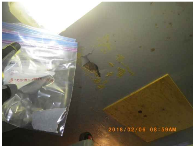
Photo 105. Sample locations LB-CS3-ACM-01A to C; grey ceiling board. Confirmed asbestos-containing material (30% Chrysotile).
