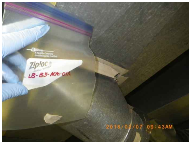
Photo 29. Sample location LB-B3-ACM-01A; paper-wrap around ducting. Confirmed asbestos-containing material (50% Chrysotile).
