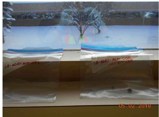
Photo 12. Sample locations LB-ADRI-ACM-05A to C; interior window caulking in hallway near R.418.
