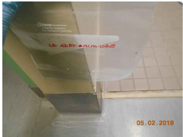
Photo 4. Sample location LB-ADRI-ACM-02B; drywall mud joint compound in R.137 (Woman's Washroom).
