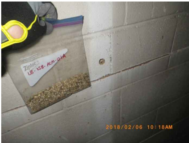
Photo 111. Sample locations LB-ISB-ACM-01A to C; wall insulation. Confirmed asbestos-containing material (1% Actinolite – Vermiculite).
