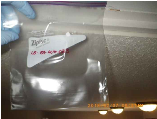
Photo 33. Sample location LB-B3-ACM-02B; textured ceiling plaster at second floor staircase. Confirmed asbestos-containing material (2% Chrysotile).
