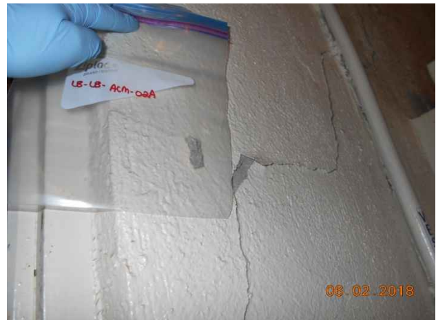
Photo 74. Sample locations LB-LB-ACM-02A to C; cement board on interior wall. Confirmed asbestos-containing material (1% Chrysotile).
