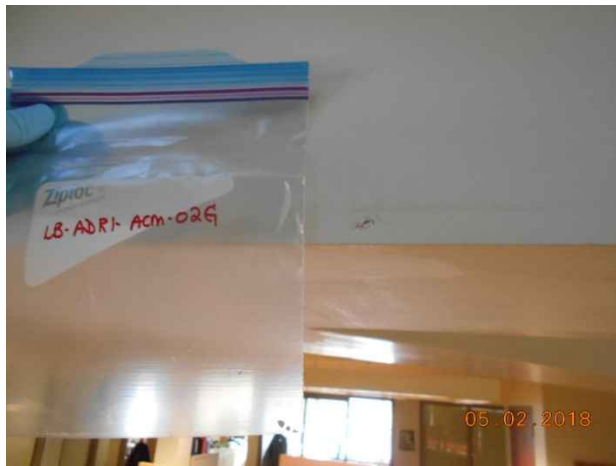
Photo 9. Sample location LB-ADRI-ACM-02G; drywall mud joint compound by front reception (Level 100).
