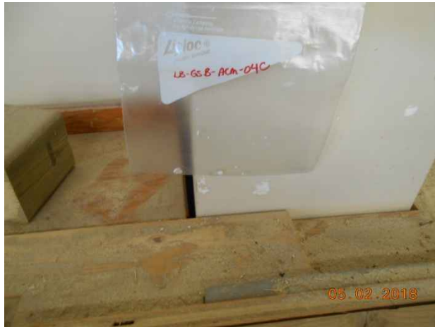
Photo 27. Sample location LB-GSB-ACM-04C; drywall mud/joint compound within the Carpenter Shop.
