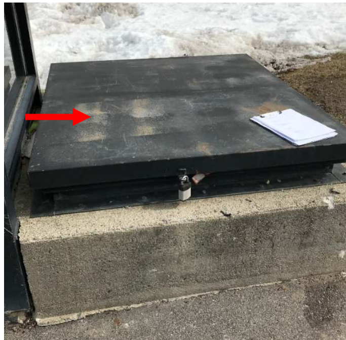
Photo 5. Manufactured black steel observed on Type H Hatch H3 is assumed to be lead-containing until bulk sampling and laboratory analysis prove otherwise. This paint could not be sampled without substrate interference.
