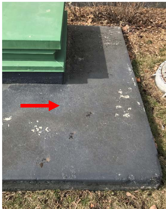
Photo 6. Black tar observed on the base of Type Q Hatch H11 was confirmed to contain 4.17% Chrysotile (DST Sample ID 1154-12A-C).
