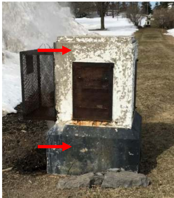
Photo 4. White paint associated with Type M Vents was confirmed to contain 5,710 ppm lead (DST Sample ID 1154-LP18). Black paint associated with Type M Vents was confirmed to contain 294 ppm lead (DST Sample ID 1154-LP19).
