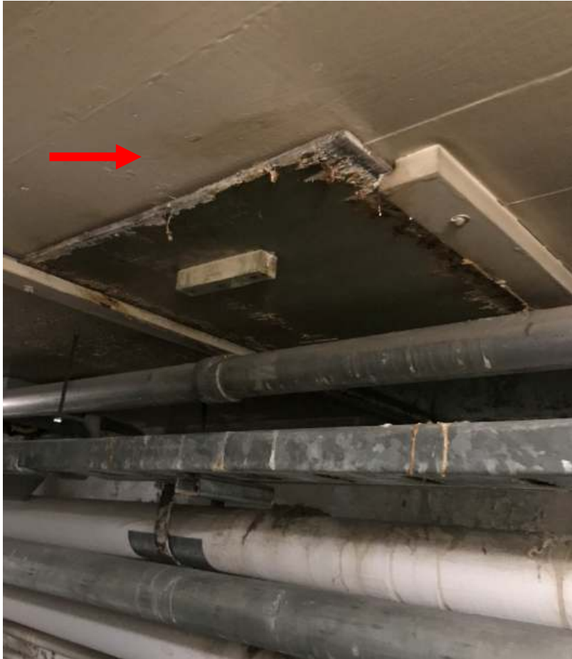
Photo 9. Grey ceiling paint within the tunnel under Type D Vent V2 was confirmed to contain 149 ppm lead (DST Sample ID 3603-LP02).
