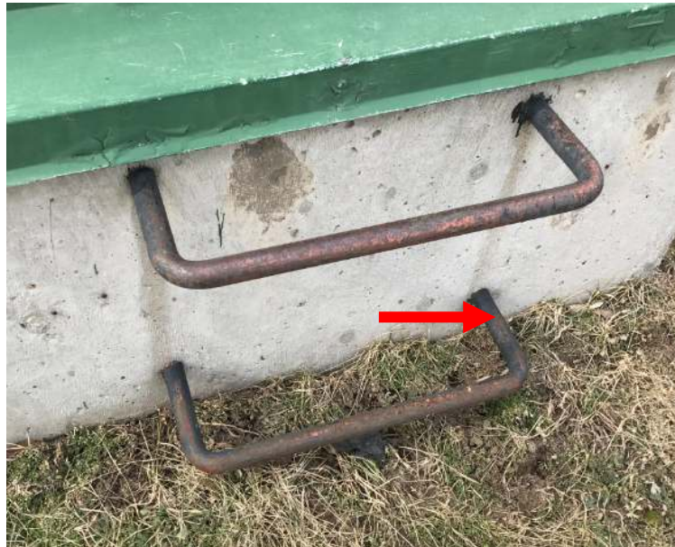
Photo 3. Black paint associated with the rebar on Type C1 Hatches was confirmed to contain 316 ppm lead (DST Sample ID 1154-LP05).
