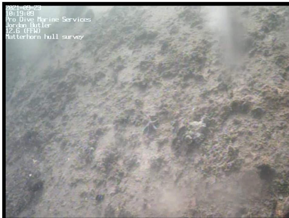
Figure 20 - Typical growth covering hull.
