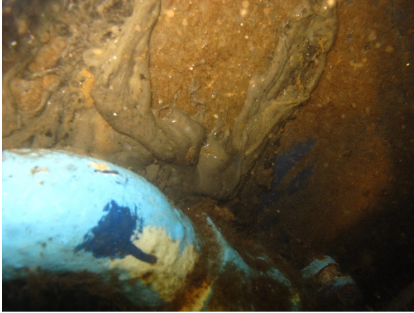
Shows slop oil by vent #2 & 4.
