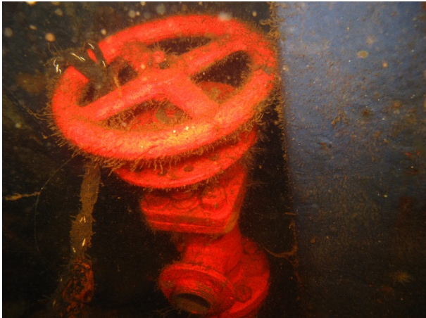
Shows gate valve in closed position.
