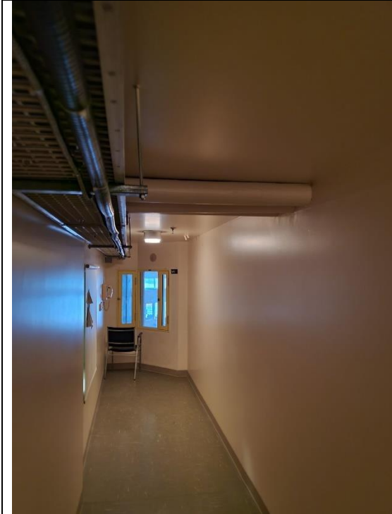
Existing ducts where it is possible to pierce the partition and have access to the suspended ceiling of the visiting department.
