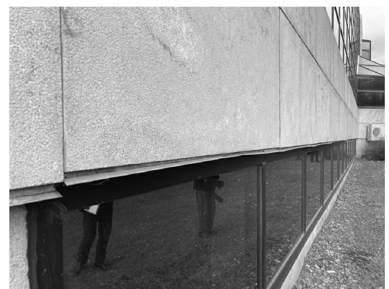
CONDITION EXISTANTE - PIERRE SUR LINTEAU STRUCTURAL / MUR-RIDEAU STONE ON STRUCTURAL LINTEL / CURTAIN WALL - EXISTING CONDITION
