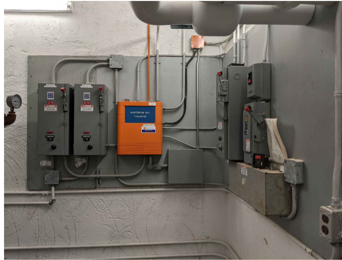
ROOM 159A - EXISTING ELECTRICAL DISTRIBUTION (VIEW #1)
