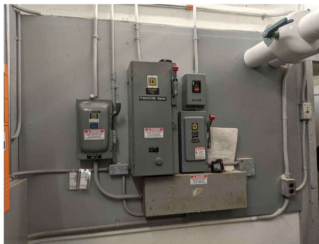
ROOM 159A - EXISTING ELECTRICAL DISTRIBUTION (VIEW #2)
