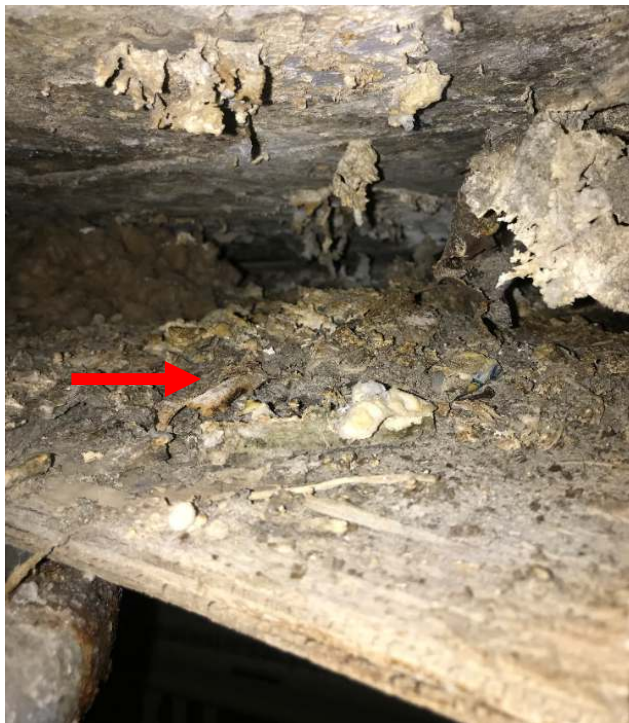
Photo 7. Miscellaneous debris observed on plywood within tunnels under the vents noted in Section 5.1.2 was confirmed non-asbestos containing (DST Sample ID 3603-01A-C to 08A-C).
