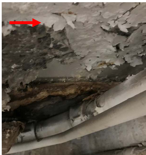
Photo 8. White ceiling paint within the tunnel under Type D Vent V1 was confirmed to contain 918 ppm lead (DST Sample ID 3603-LP01).
