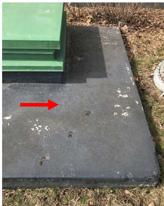
Photo 6. Black tar observed on the base of Type Q Hatch H11 was confirmed to contain 4.17% Chrysotile (DST Sample ID 1154-12A-C).
