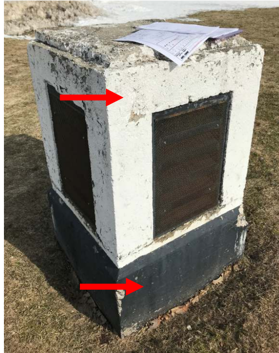
Photo 1. White paint associated with Type D Vents was confirmed to contain 622 ppm lead (DST Sample ID 1154-LP01). Black paint associated with Type D Vents was confirmed to contain 176 ppm lead (DST Sample ID 1154-LP02).
