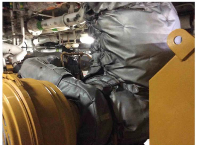
40 Material sample Engine Room — Pipe — Canvas — Fair — Asbestos-free material Chantal.Soulard - 2022-02-07 16:23
