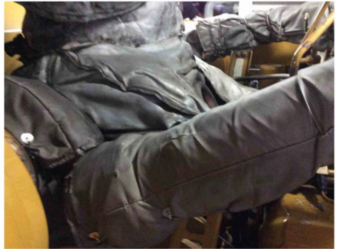
39 Material sample Engine Room — Pipe — Canvas — Fair — Asbestos-free material Chantal.Soulard - 2022-02-07 16:21
