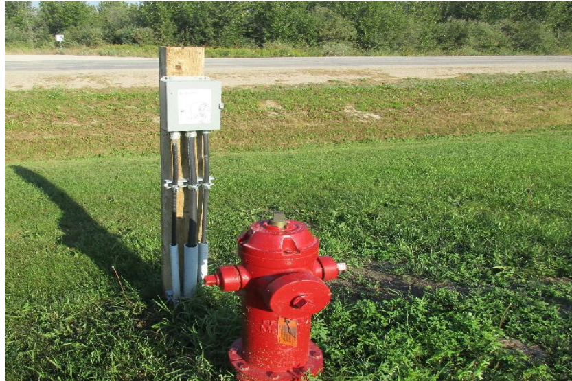
G3011 - Underground Water System - Hydrant
