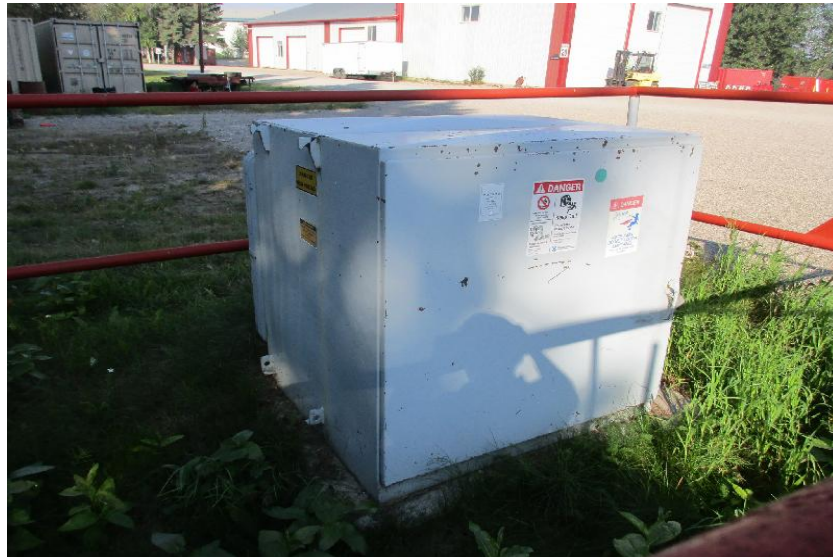
G4013 - Underground Electrical System - Service Transformer
