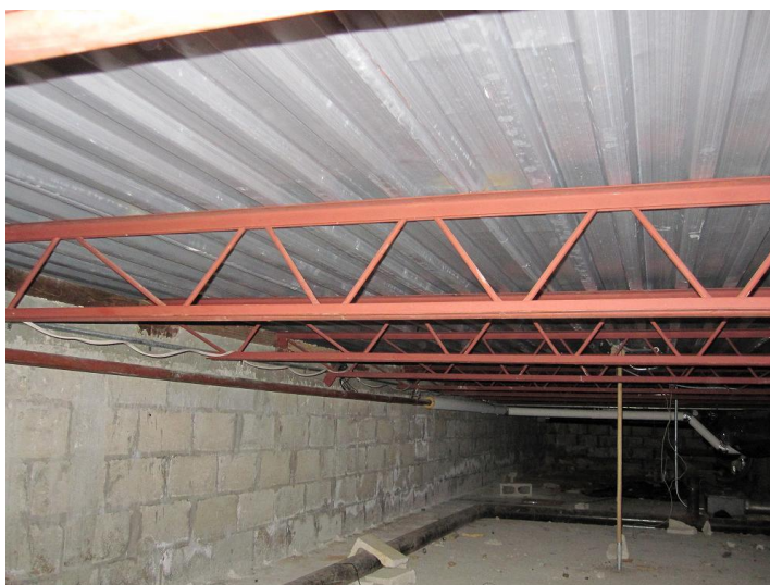
Photograph No. 2 - Basement Foundation Wall Efflorescence
