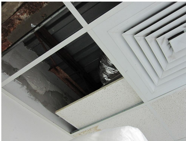
Photograph No. 4 – Basement Level Member Corrosion
