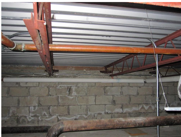
Photograph No. 1 – Basement Foundation Wall Efflorescence
