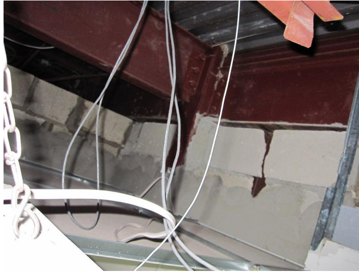
Photograph 7: Unsupported Concrete Masonry Partition Wall
