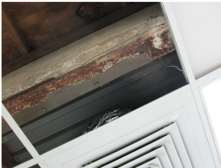
Photograph No. 3 – Basement Level Member Corrosion
