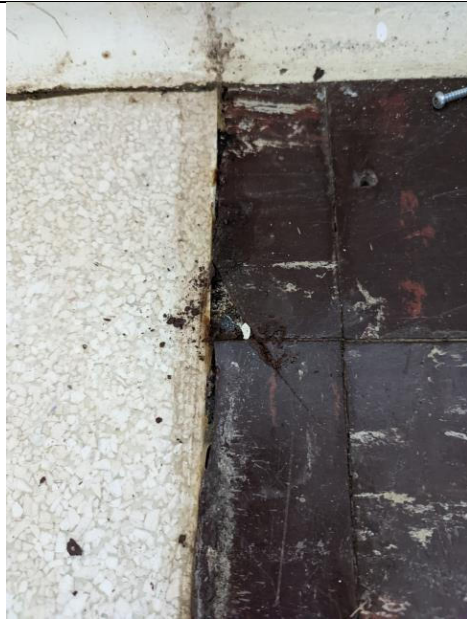
Sample: 38686 - 12 Location: Building 12, Room 13 Description: Vinyl Floor Tile Asbestos: 3% Chrysotile
