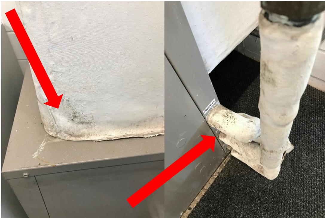
Photo 3&4: Suspected mould observed on the ductwork and associated piping (non asbestos insulation) outside of room 201.
