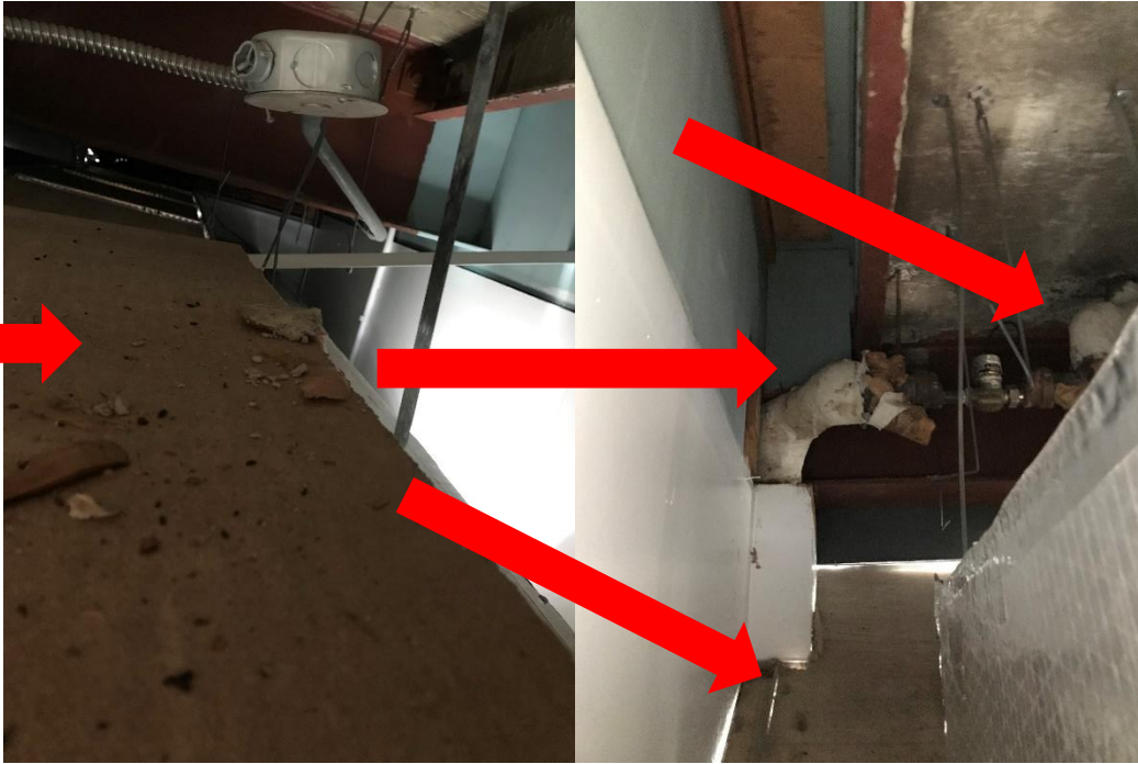
Photo 1&2: Four grey cement compound fittings in poor condition observed on the steam pipe concealed behind the wall in the corner of the room near the window in room 201 was confirmed to contain 40% Chrysotile asbestos (Englobe Sample ID M-46-02A). Approximately one square metre of debris was observed on top of ceiling tiles near the pipe in the bulkhead. Rodent fecal matter was also observed on the bulkhead ceiling tiles.
