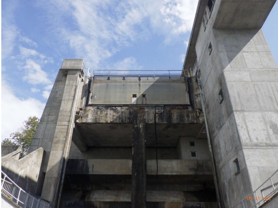
Photo 3. North Chamber Upper Reach Gate.
