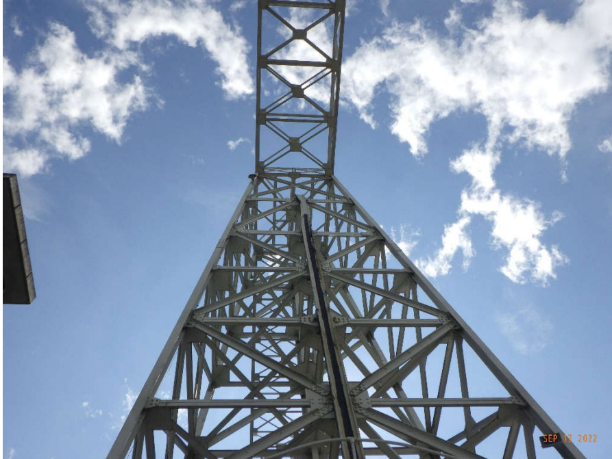
Photo 1. North Chamber South Guide Rail.
