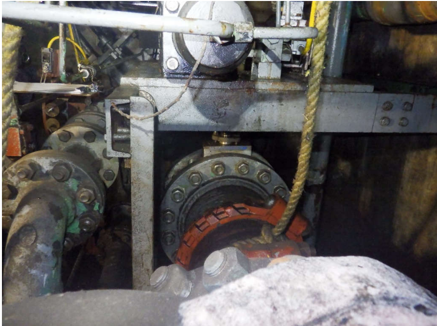
Photo 10. Cross-Over Valve. Cross-Over Pipe is 12 Inch NPS.
