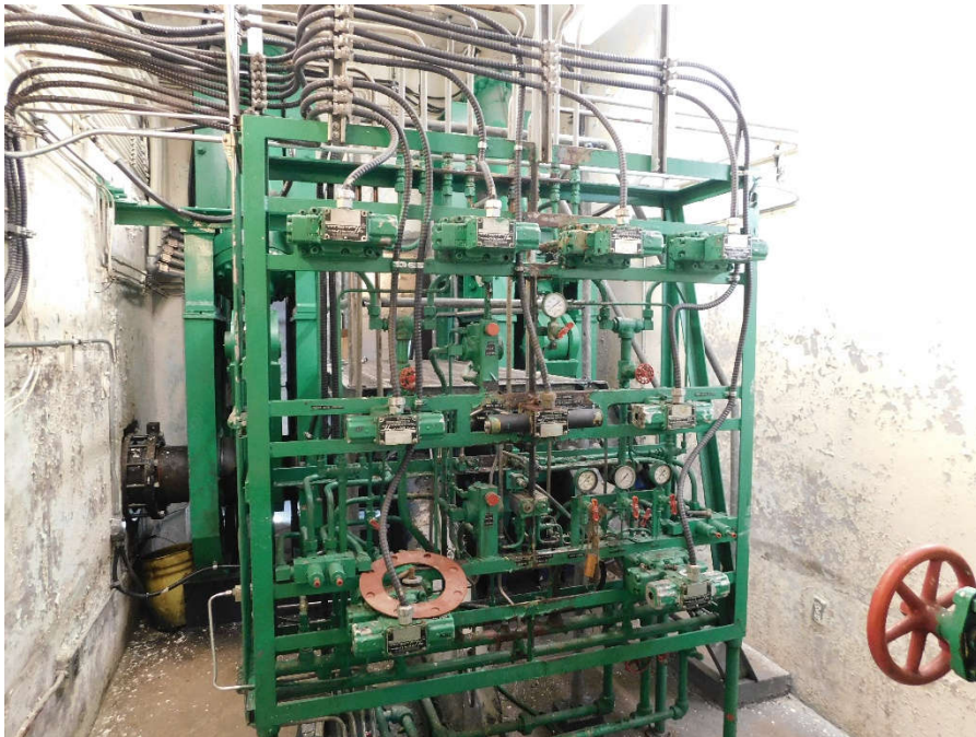
Photo 8. Hydraulic Valve Rack, Typical of Multiple Location at Site.
