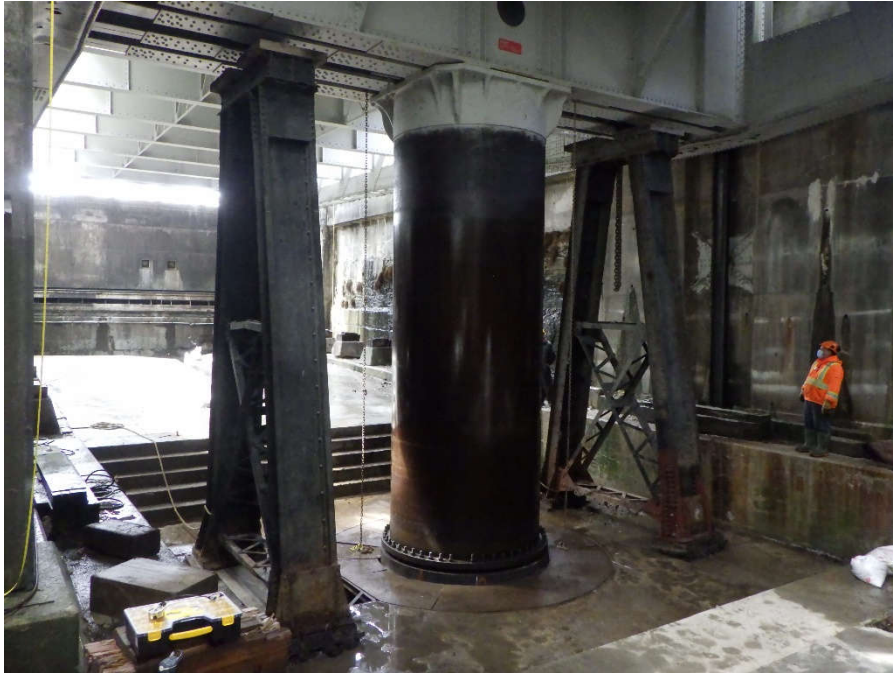
Photo 7. Chamber on Support Stands for Winter Layup. Note Ram Diameter 90 Inches.
