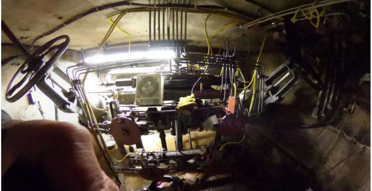
Photo 9. Cross-Over Valve and Isolation Valve Room. (Permit Required Confined Space)
