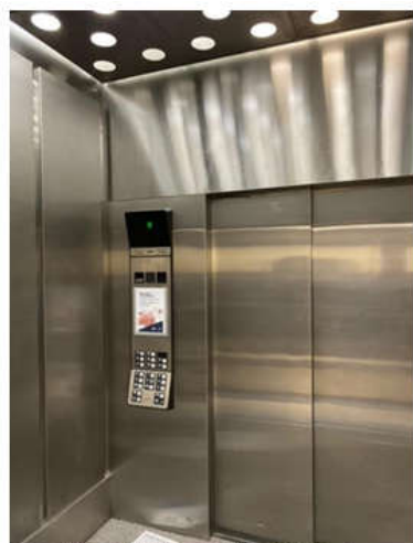
Picture 5: Picture inside freight elevator
