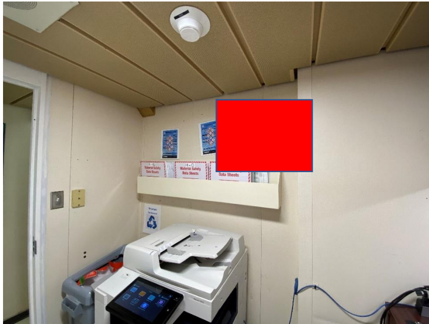
Figure 18.4-2: Location of new cabinet in the Photocopier Room (225)
