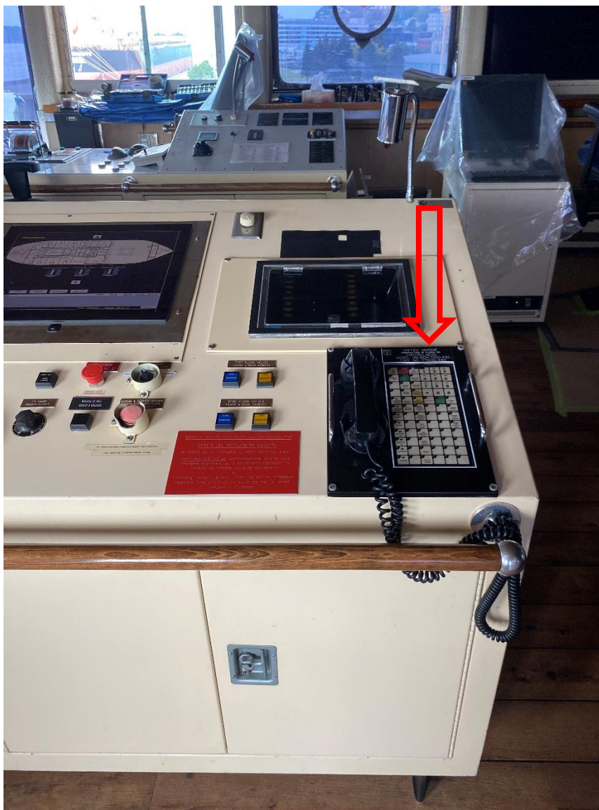
Figure 18.1-1: SICS Control Head in Wheelhouse
