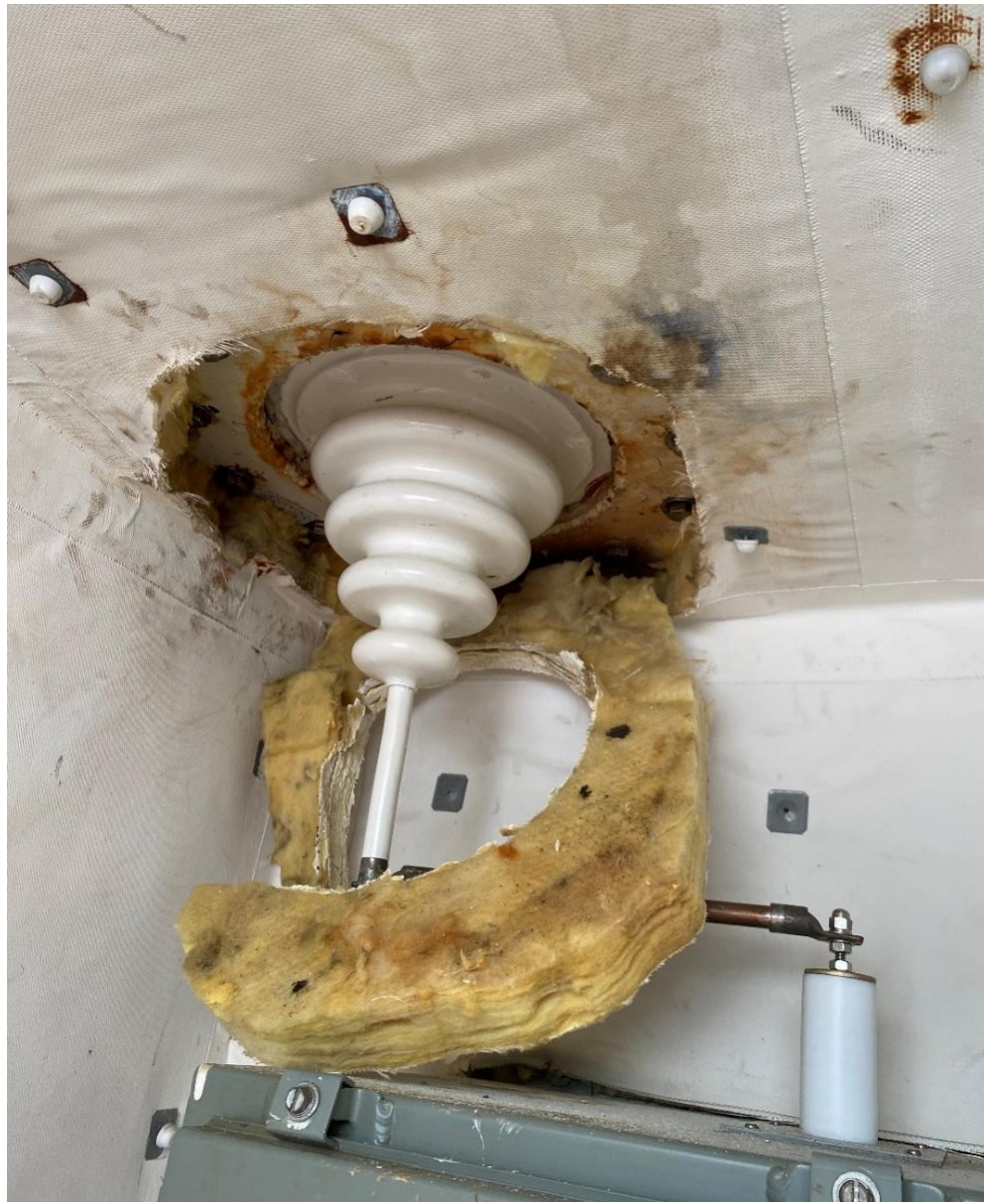
Figure 18.8-6: Existing ATU Isolator
