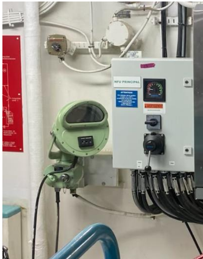
Figure 18.2-10: Existing repeater in Steering gear compartment
