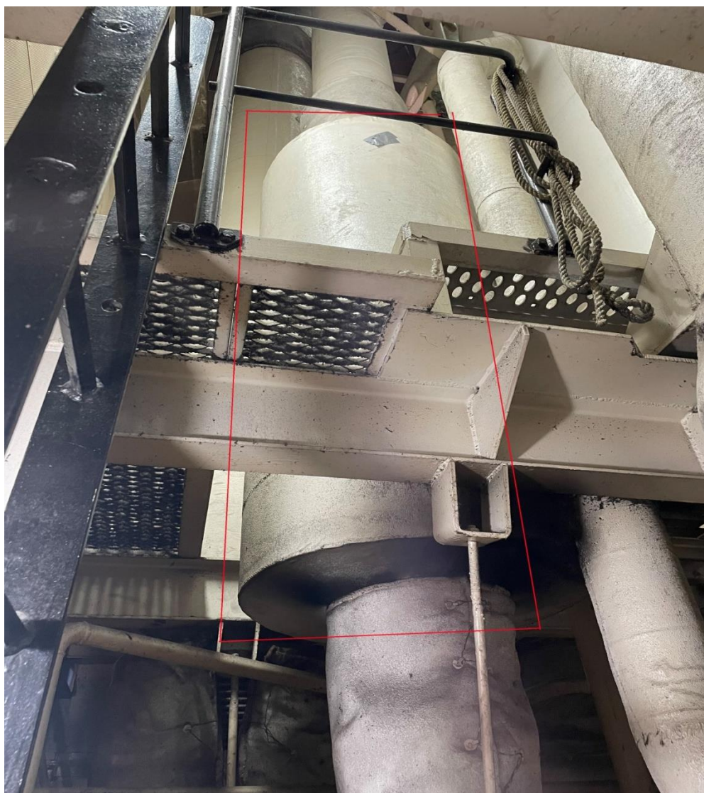
Figure 13.2.1 Auxiliary generator silencer
