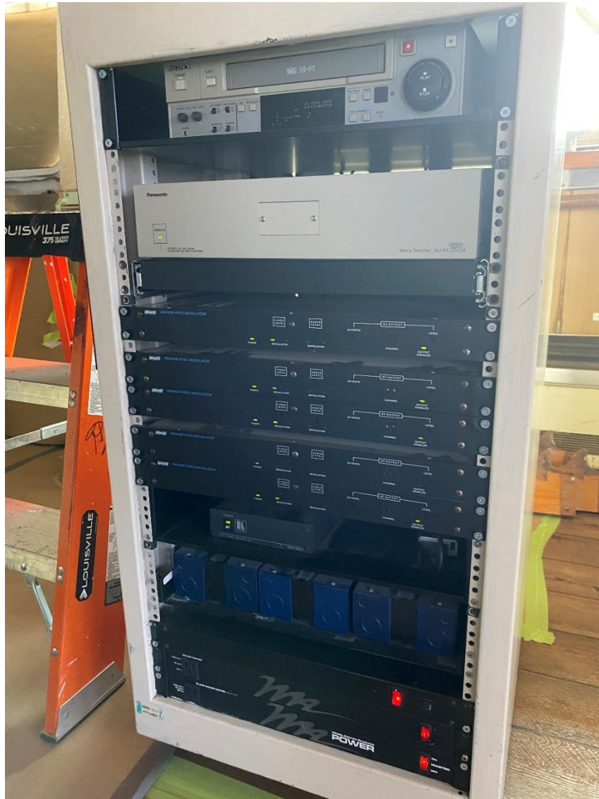
Figure 18.6-2: Front of CCTV Cabinet
