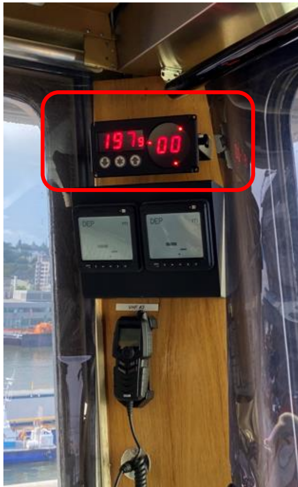
Figure 18.2-2: Existing Digital Repeater to retain
