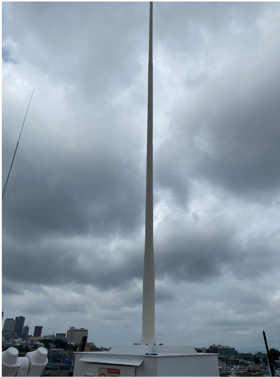
Figure 18.8-1: NDB Antenna on top of the enclosure
