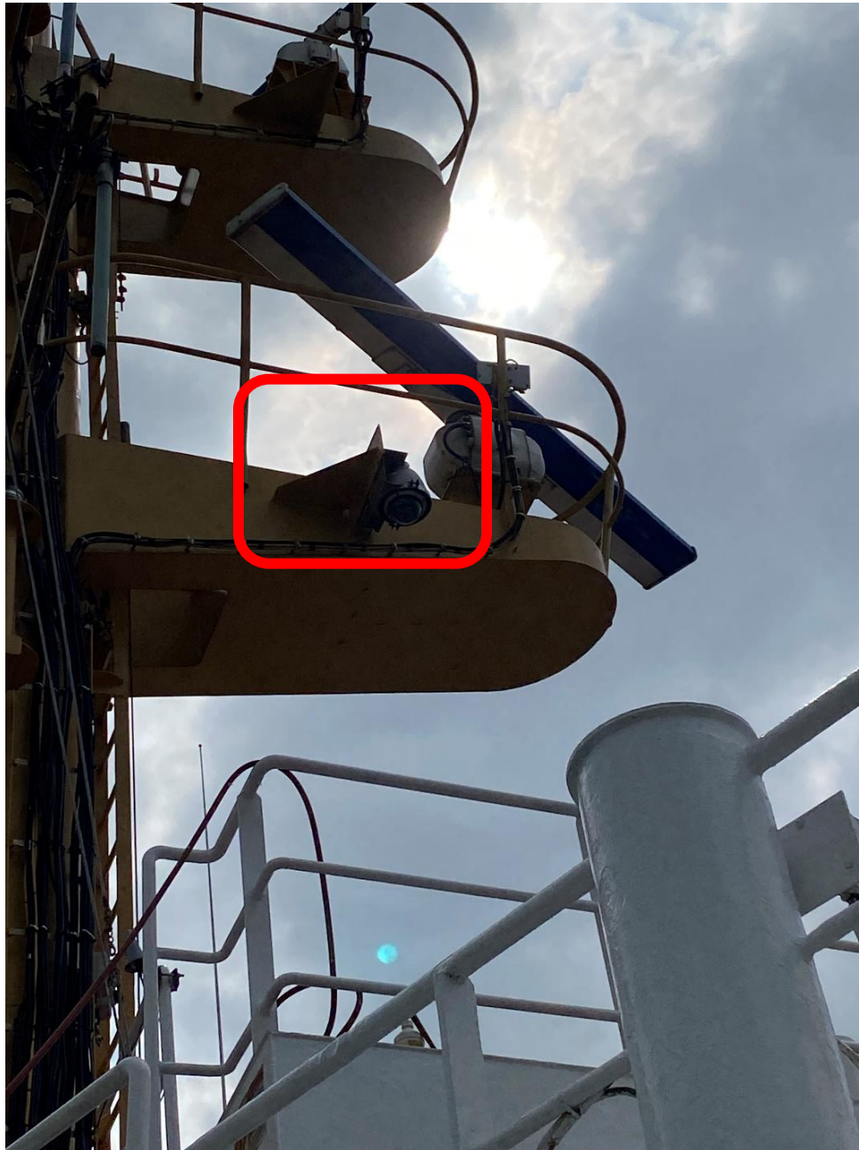
Figure 18.6-5: FWD Mast camera to be replaced
