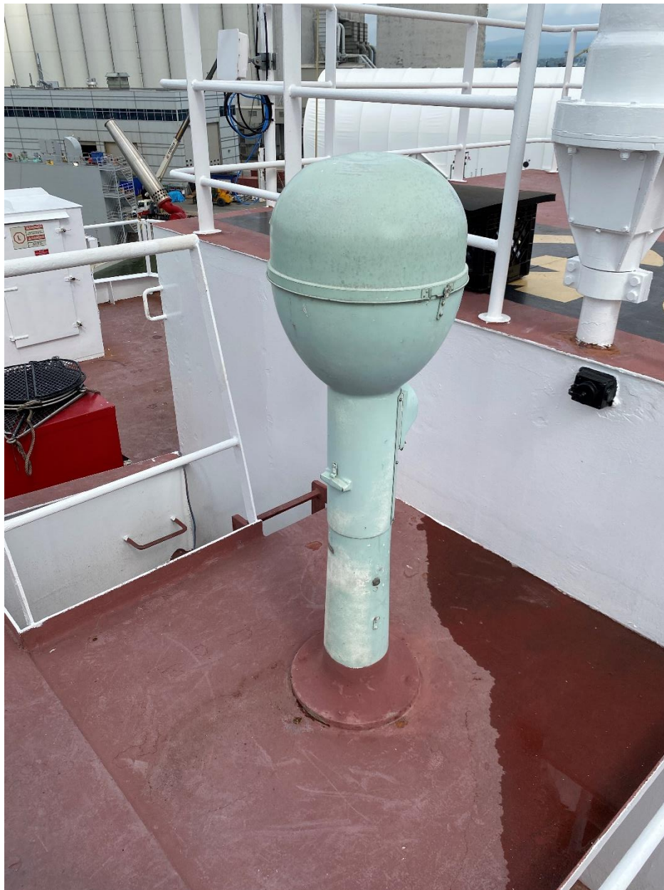
Figure 18.2-6: Bearing repeater on stand (Top of wheelhouse)
