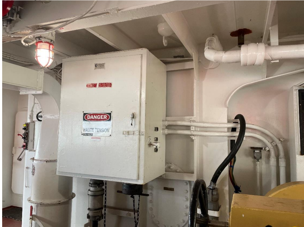
Figure 11.6.5 Shore power electrical panel
