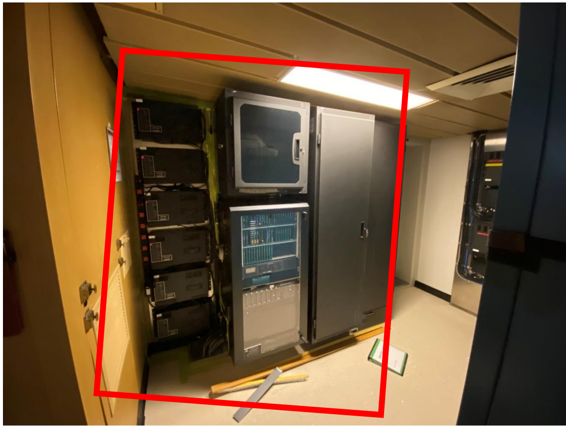
Figure 18.1-2: Existing PA and Talkback Cabinets and Amplifiers
