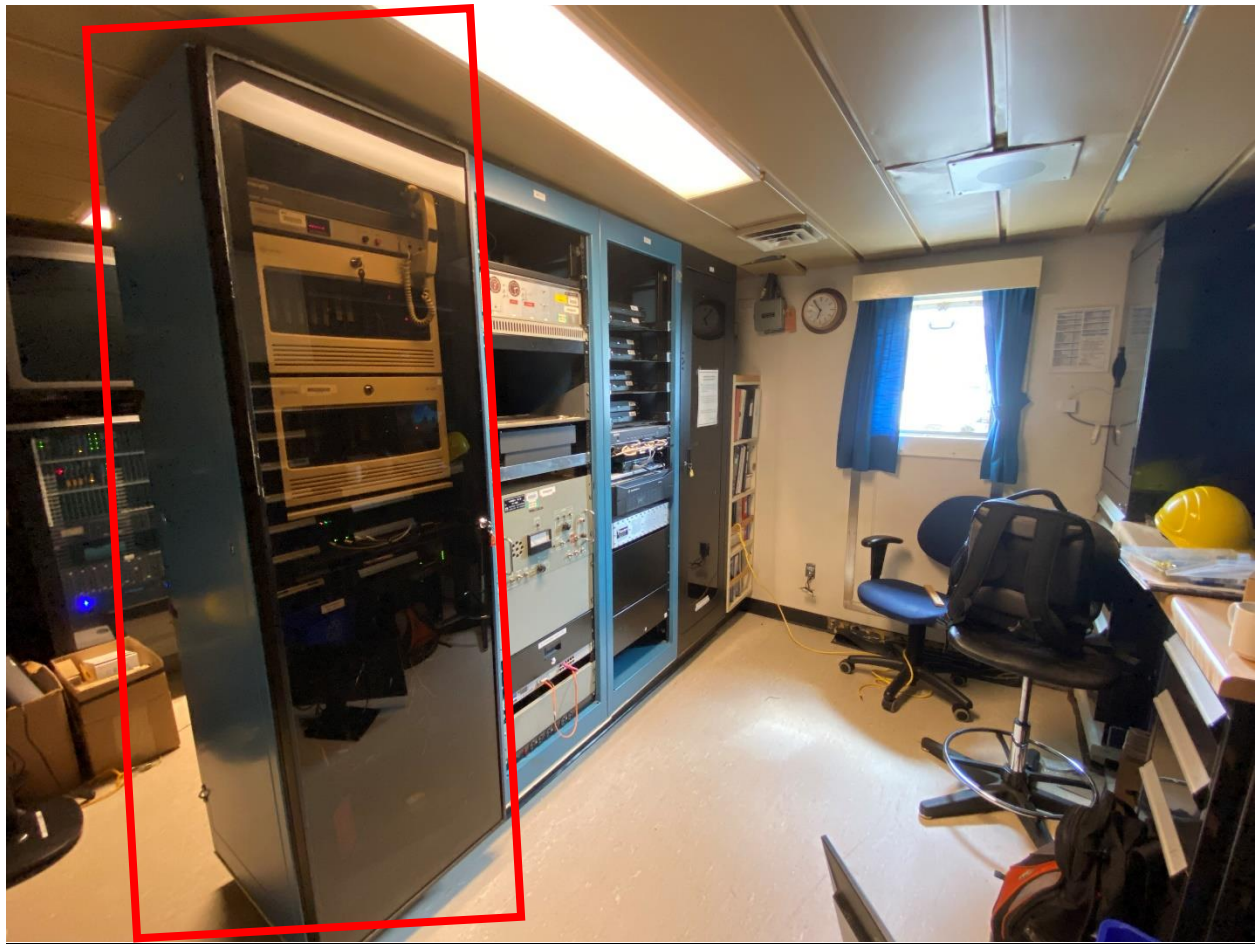
Figure 18.1-3: Existing Telephone System Cabinet (Rack #3)
