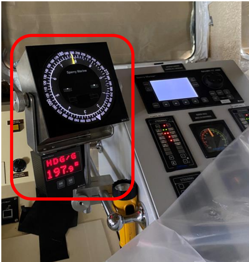
Figure 18.2-1: Existing helm position repeaters to retain
