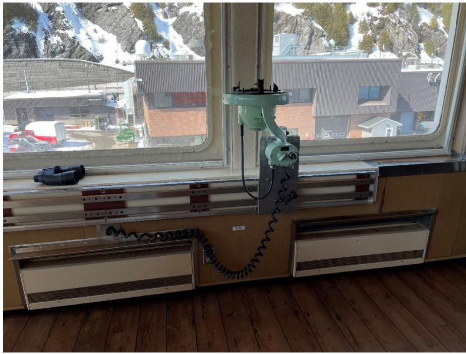
Figure 18.2-9: Bearing Repeater on sliding rail (Stbd side)
