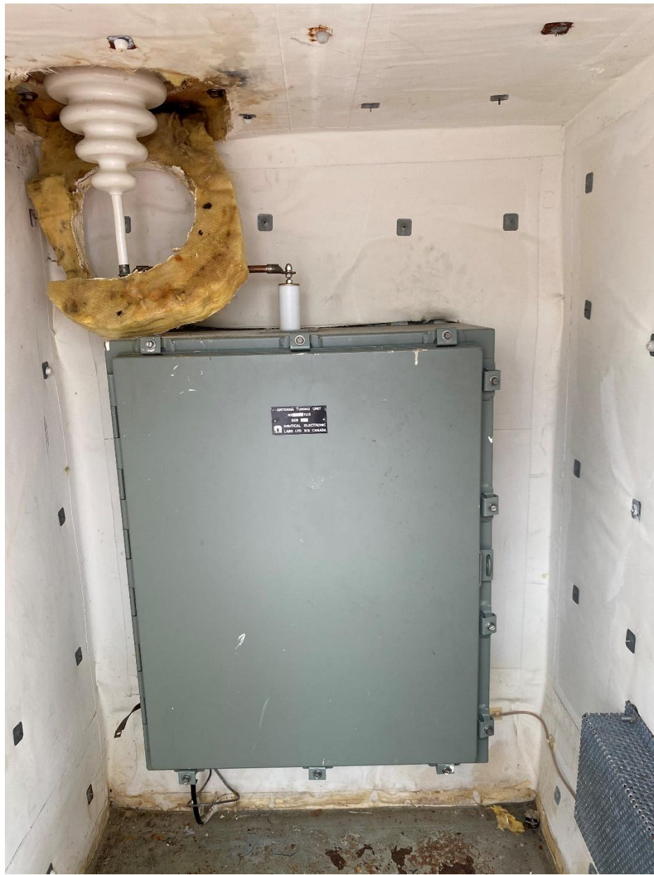
Figure 18.8-5: Existing NDB ATU to be removed
