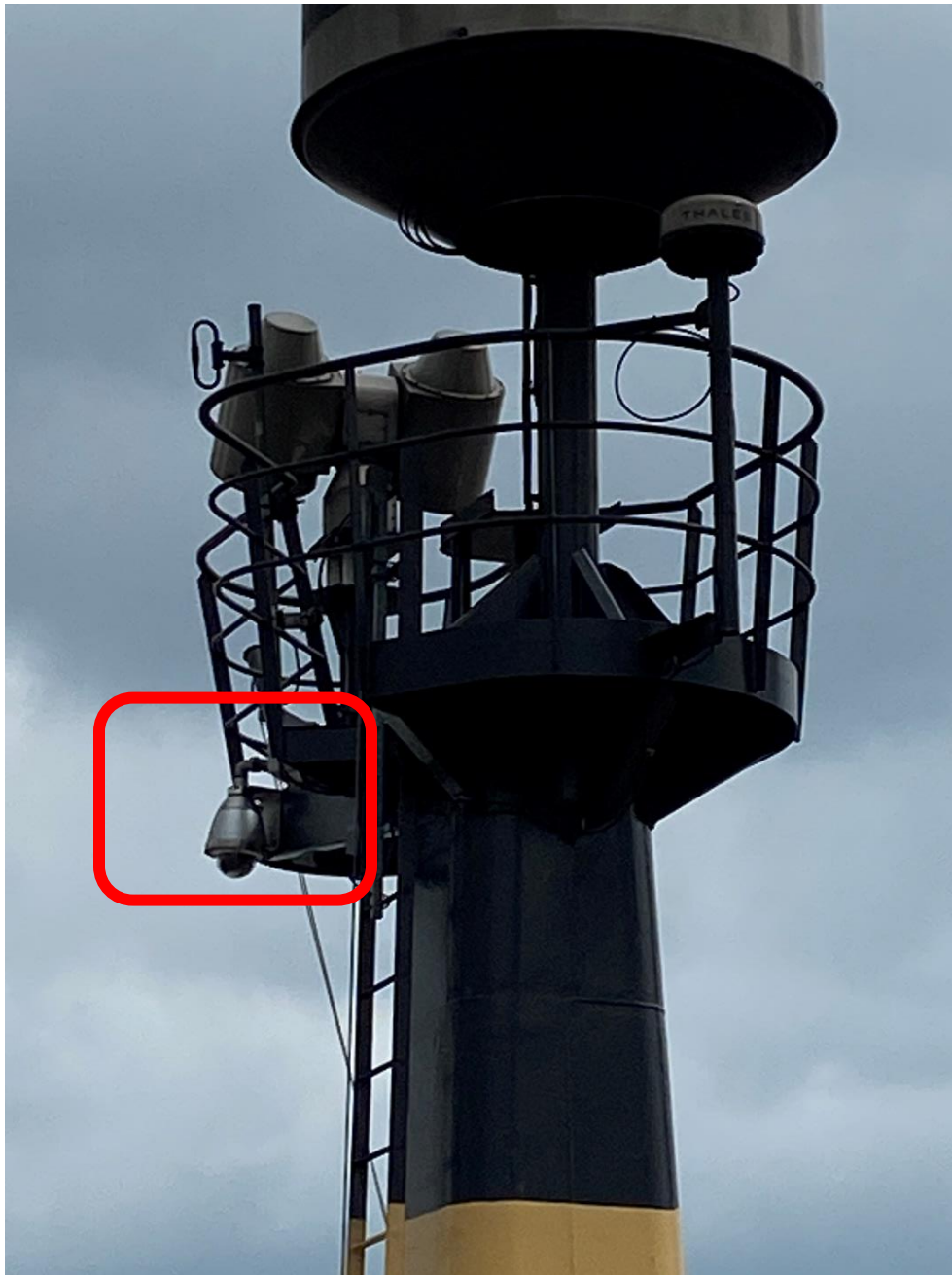
Figure 18.6-6: AFT Mast camera to be replaced
