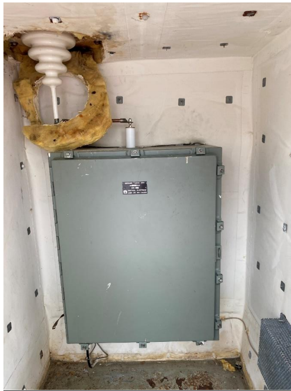
Figure 18.8-2: NDB ATU Inside enclosure
