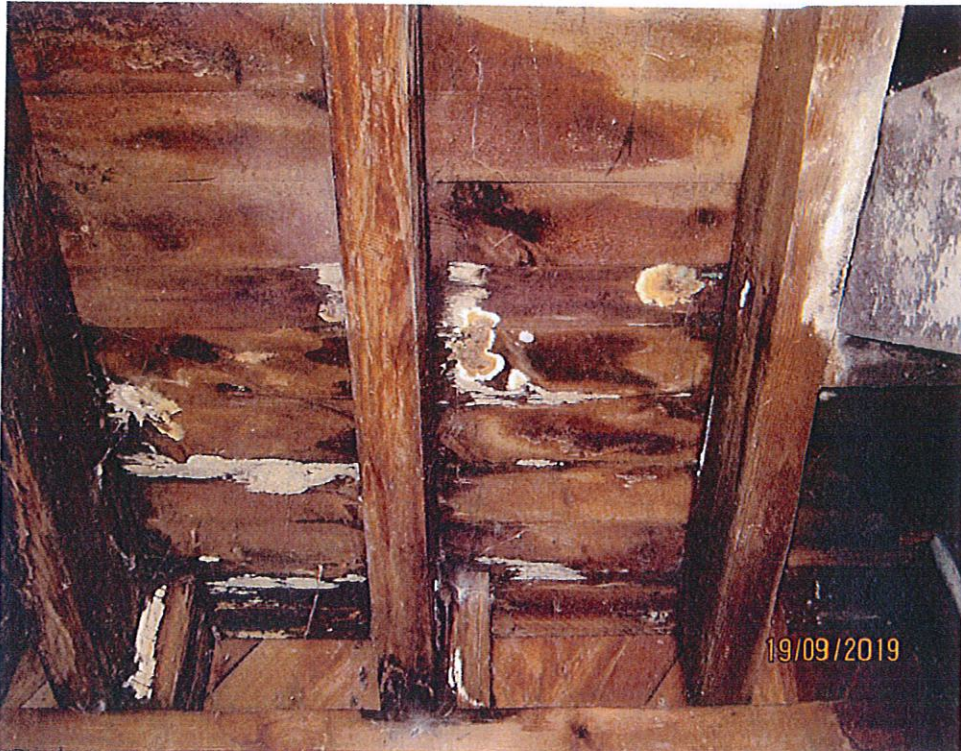
Photo 7: Visible indications of fungal growth on the ceiling of the 1 st level.
