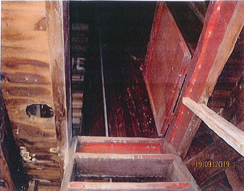
Photo 9: View facing up from the 1 st level ladder staircase. More red paint is visible.
