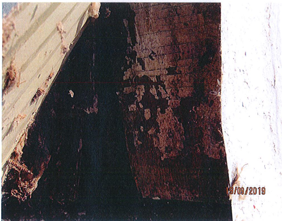
Photo 2: View of the white painted shakes located under the metal exterior sheeting. This paint contains a lead content of 50,000 mg/kg.
