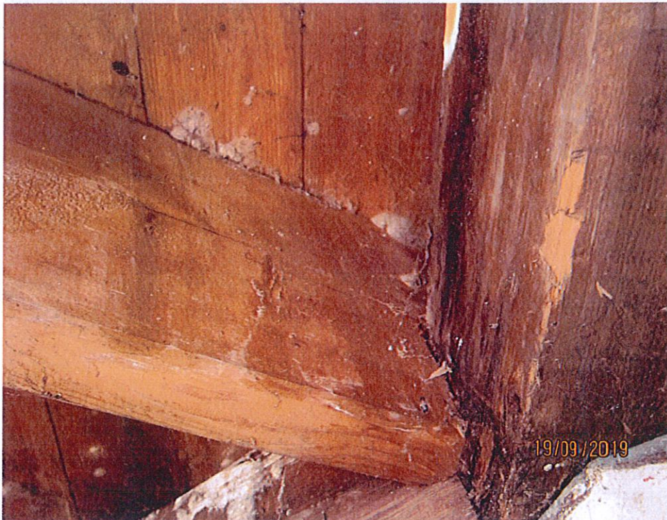
Photo 10: Visible signs of fungal growth on the 2 nd level.
