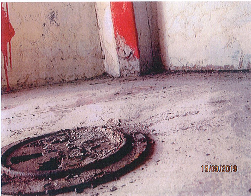
Photo 12: View of a floor vent and metal covered flooring on the 3 rd level.
