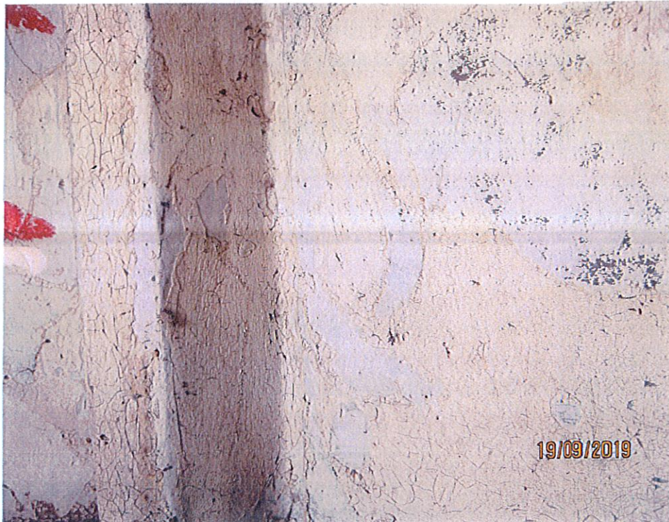
Photo 11: The walls of the 3 rd level contained similar white paint as the shakes.
