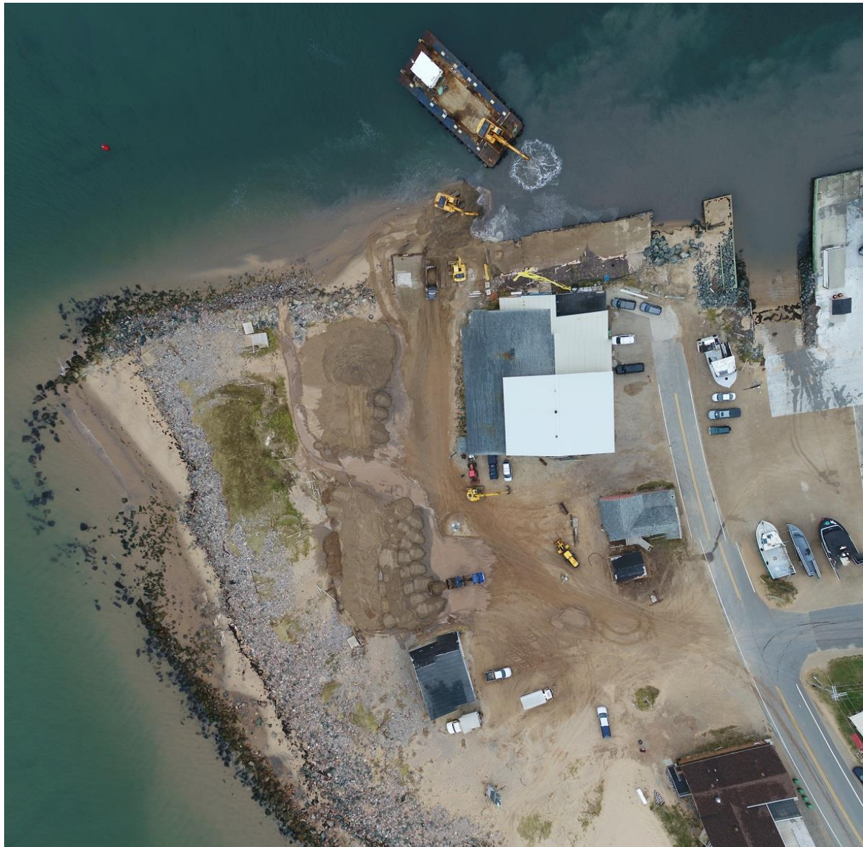
Figure 2.1 Composite photo of the western sector of the fishing harbour (dredging operation in progress)
