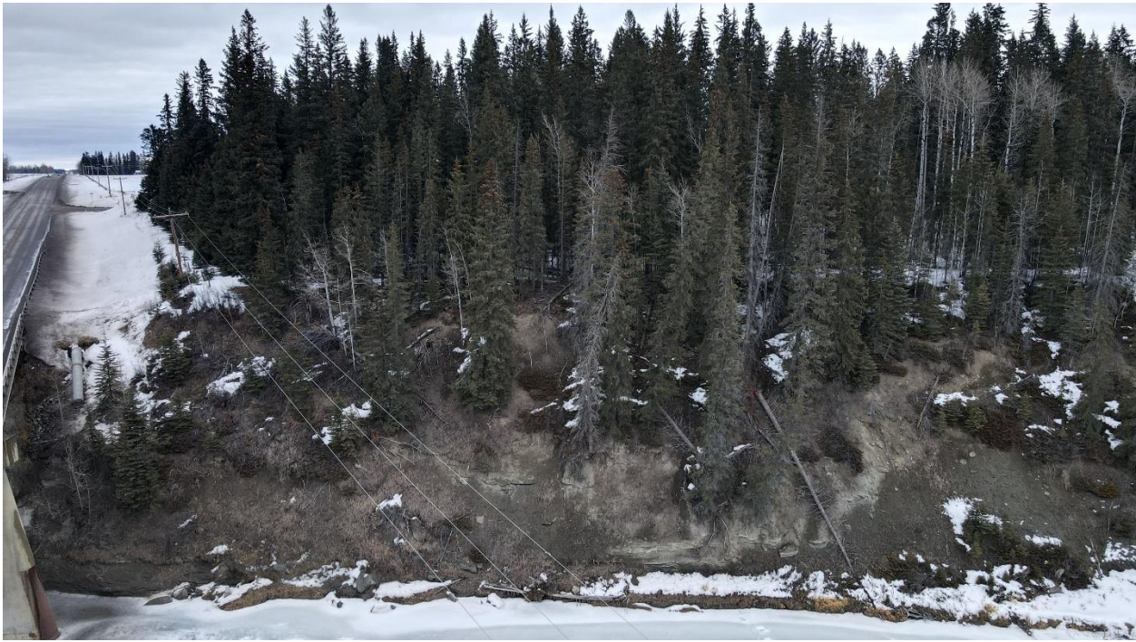
Figure 3: Aerial View of Right Bank Far Side from Left Bank Home Side
