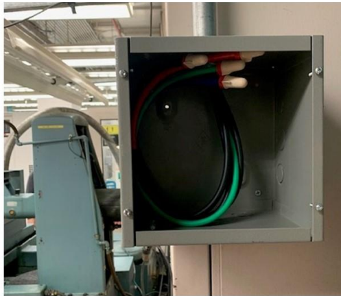
208 VAC / 3 Phase / 60 Hz, 70 amps power supply
