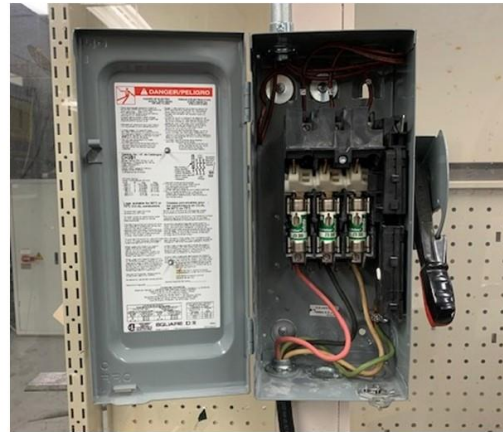
575 VAC / 3 Phase / 60 Hz, 30 amps power supply
