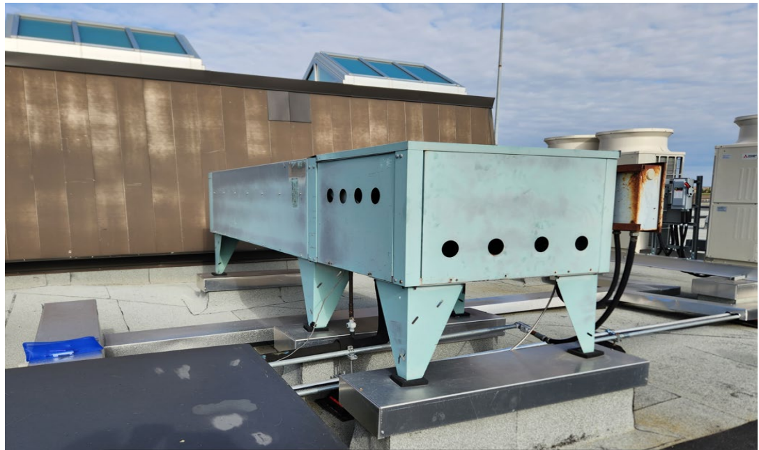
Photo 2: Cooling unit to be replaced
