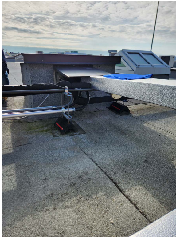
Photo 3: Roof box for refrigerant piping.
