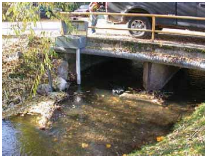
Figure C-10. The deployment tube must protect the sensors from debris, such as leaves and branches, in the stream. Photo: Linda Gregory
