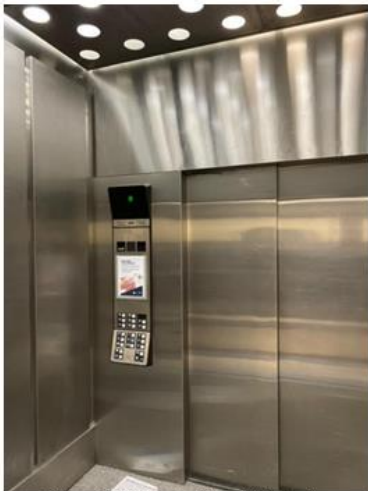
Picture 5: Picture inside freight elevator
